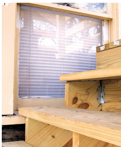
Figure 8. Safety glazing must be used near stairs.
