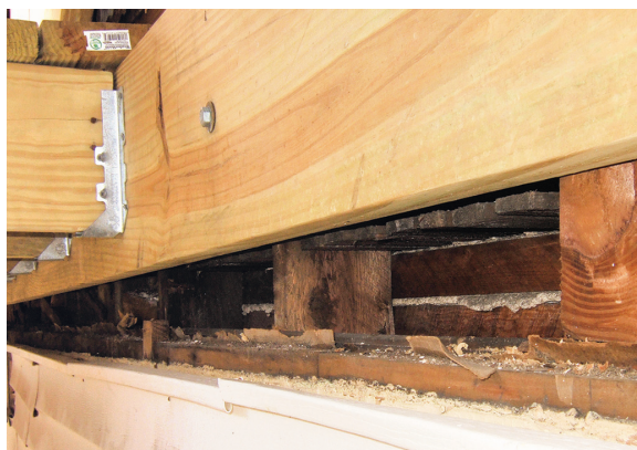
Figure 2. Required flashing and sheathing behind the deck ledger are missing, and the bolting schedule appears to be inadequate.
