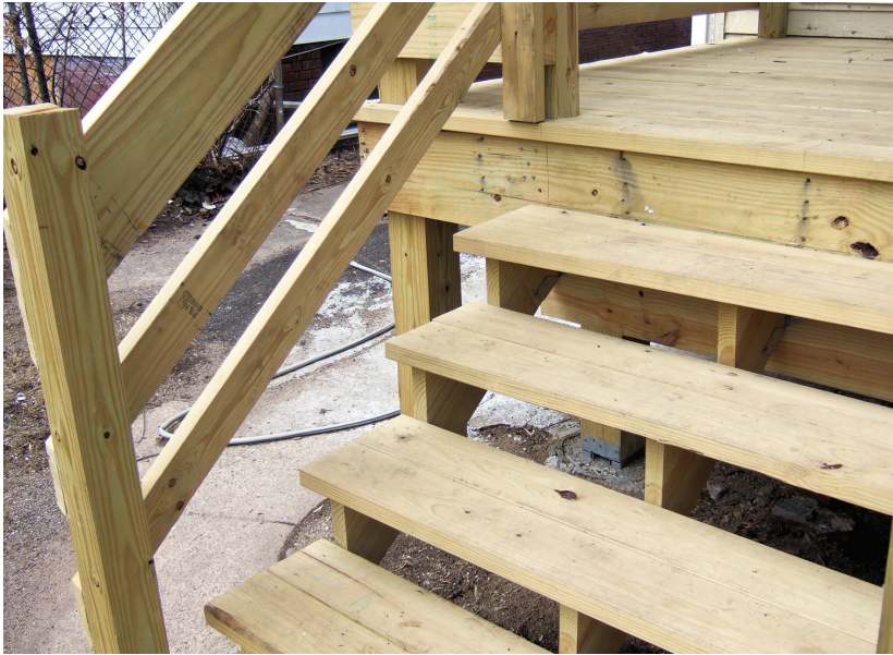
Figure 9. On notched stairs, the space between the bottom guard and the rear of the treads must be no larger than 6 inches.
