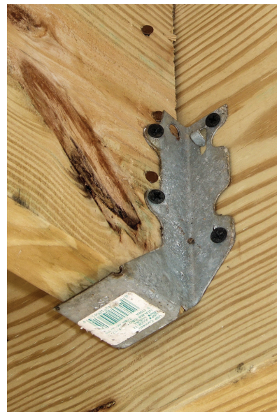
Figure 3. Drywall screws lack both the shear strength and the corrosion resistance to be used as structural deck fasteners.
