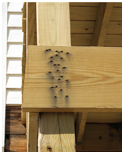
Figure 5. Non-corrosion-resistant nails are inadequate for this connection, no matter how many are used.
