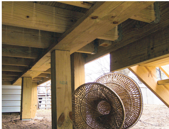
Figure 1. Even with concrete footings below, a 2x8 on the flat does not qualify as a beam.
